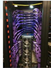
Neat Rack Wiring
